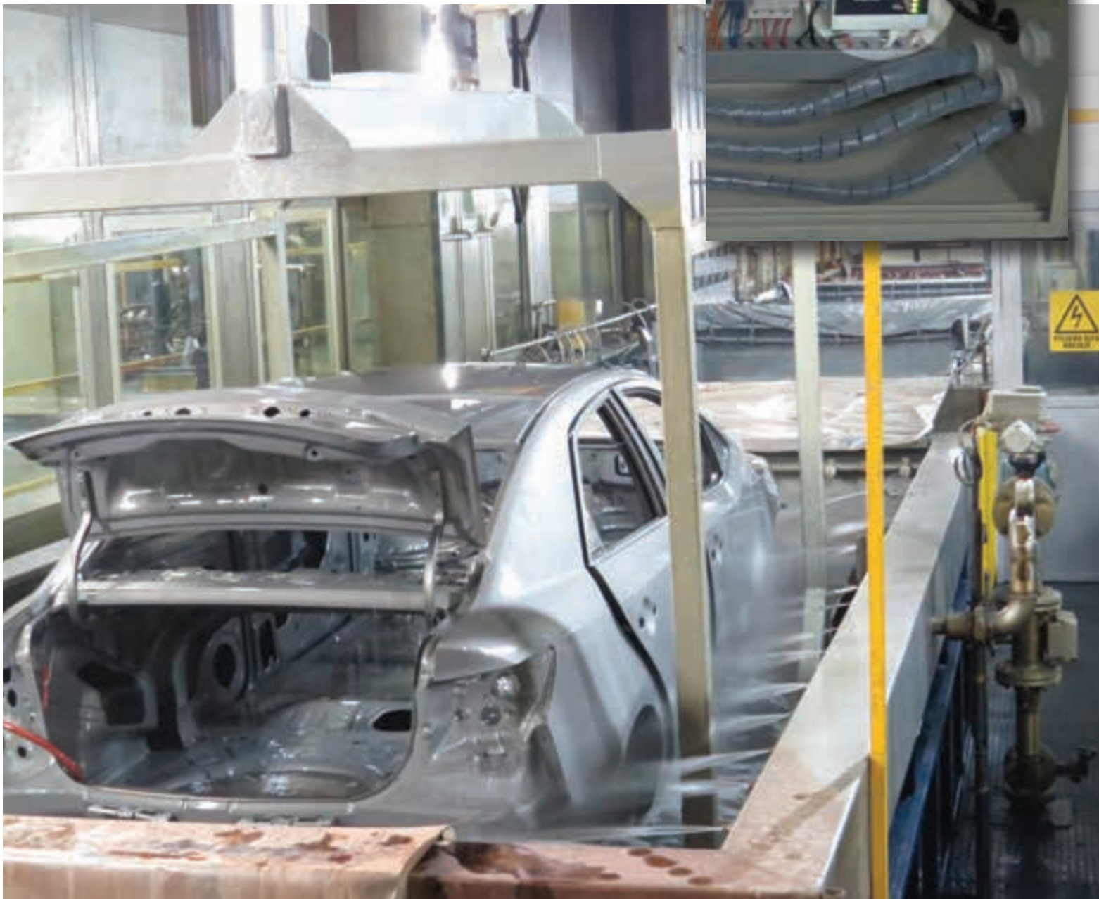
Collisions between mobile carriers were reduced by 100% with the installation of ProSoft Technology® radios.
