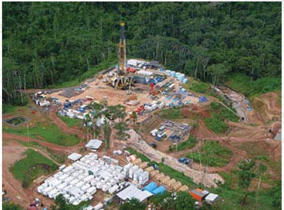
Most of the equipment needed for the Camisea project was flown in and lowered from the air onto hilltop clearings.
